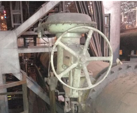
Before - Poor Control with Pneumatic
