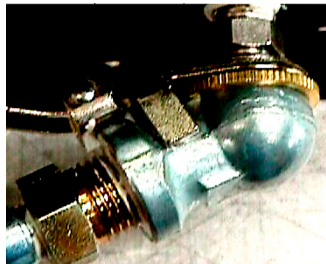
Figure 1.6.4-6 Fill Valve with Schrader fitting.
