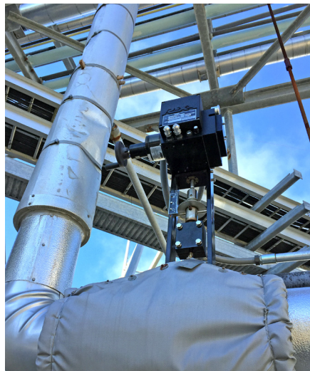
Steam to Fuel Gas Heater
