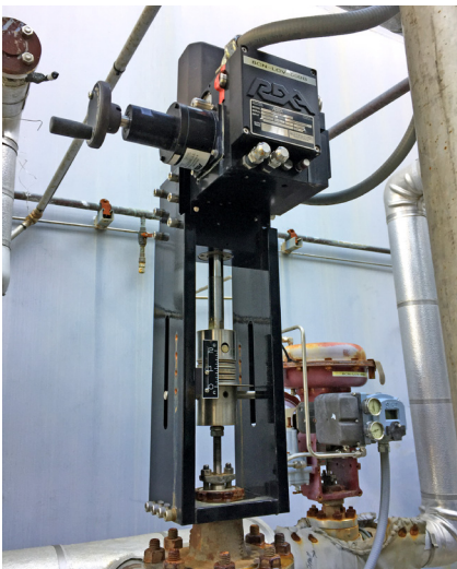
Condensate Level Control
