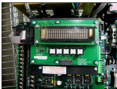
Photo 4.E.12.2-2 Internal VFD Display Assembly
