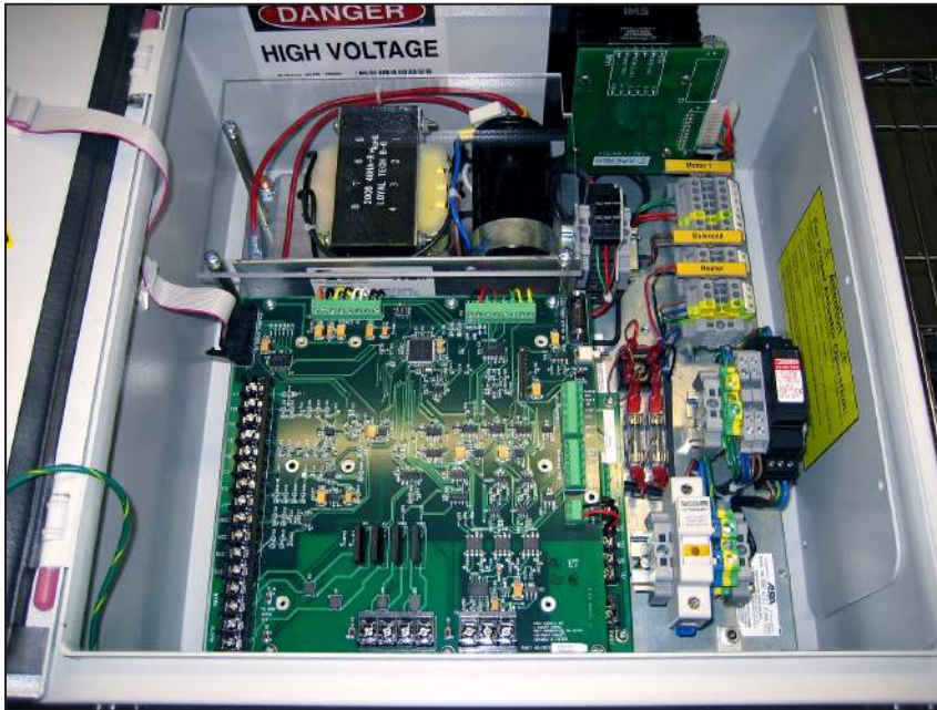
Photo 3.2 B stepper driver external power supply
