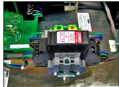
Photo 4.E.12.4-2 Input and output wires
