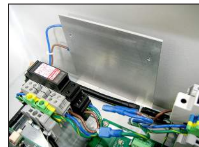
Photo 4.E.15.1-5 Bracket, filter removed
