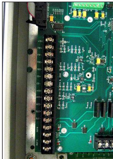
Photo 4.E.4.1-4 TB1 Connections Terminal
