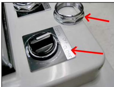
Photo 4.E.18.1-5 Switch label and bolt
