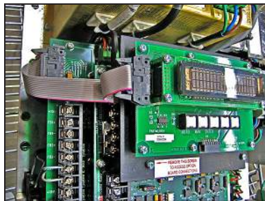
Photo 4.E.11.2-1 Internal VFD Display Assembly
