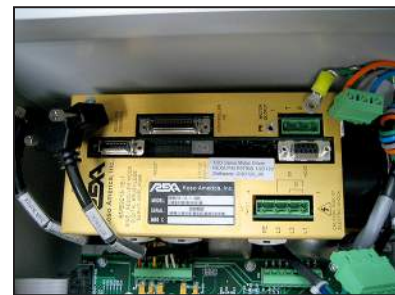
Photo 4.E.9.1-2 Servo drive cable connections
