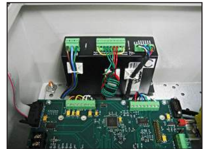
Photo 4.E.6.1-1 Stepper Motor Drive
